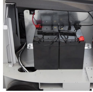
Separate gates, one for charging battery and general maintenance
